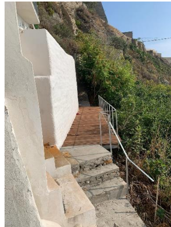
The Wall of Migrants, vicolo San Domenico, Procida Work in progress – September 2021
